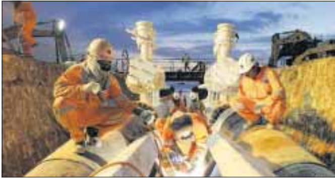
Cairn Energy workers build a pipe in India as the oil explorer posted a surge in profits. The company reported pre-tax profits for the first half of 2011 of £733million, compared with £88million in 2010. Shares in Cairn and its rivals rose on the prospect of Libyan oil returning to the market Picture: PA
